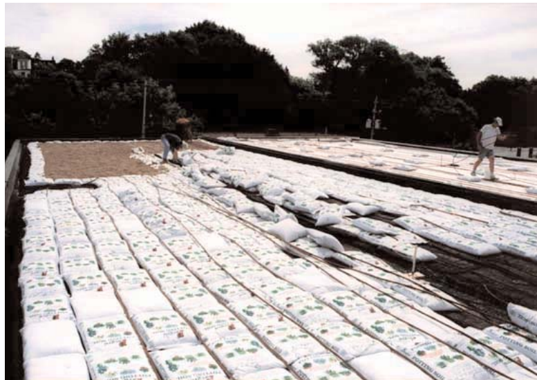
Installation of the Garland GreenShield™ and the Soprema Sopranature™ green roof systems.
