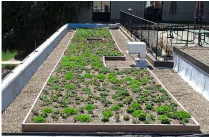
A green roof by Garland on a nursing home
